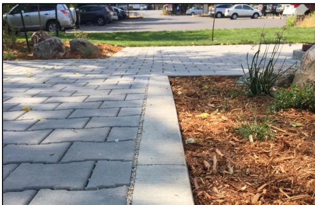
Figure 5.4-6. PICPs with Perimeter Barrier Source: Courtesy of the City of Bozeman
