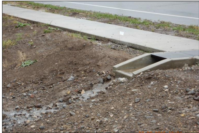
Figure 5.6-6. Degrading Concentrated Flow Inlet Source: HDR
