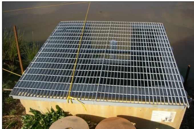
Figure 5.8-5. Outlet Structure Trash Rack
