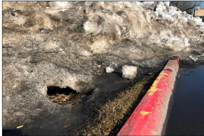
Figure 4-4. Snow on Storm Drain Inlet
