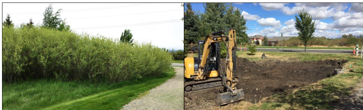
Figure 5.7-6. Detention Basin Deferred Maintenance
