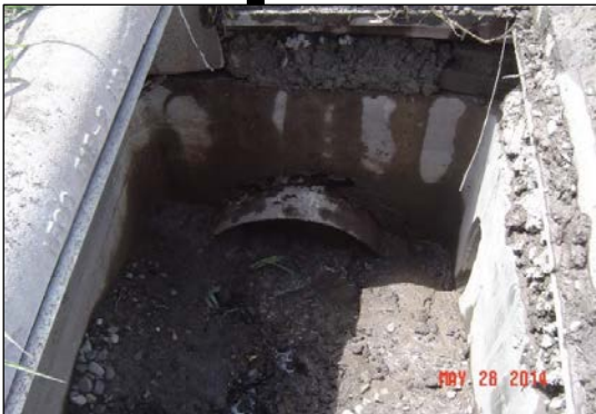
Image 3 - Clogged stormwater inlet from construction
