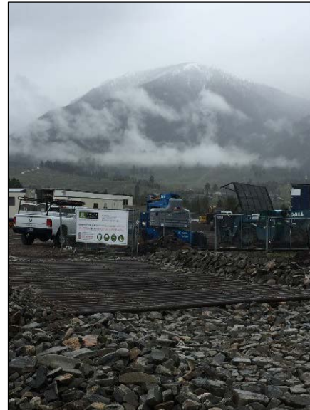
Image 24 - Properly installed cattle guard/angular rock hybrid entrance
