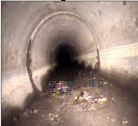
Image 1 - Clogged stormwater pipe from construction
