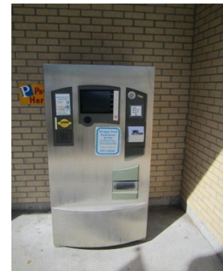
Existing Bridger Garage Pay Station
