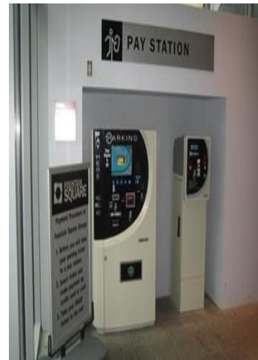
Example: Pay on Foot in elevator lobby – Fountain Square Garage, Cincinnati OH
