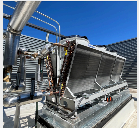
Rooftop heat pump unit at Fire Station #2
