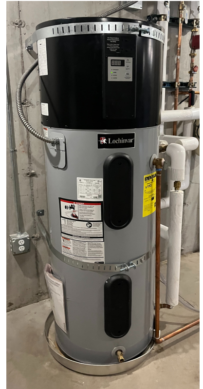
HPWH installed at the Bridger View Development in Bozeman
