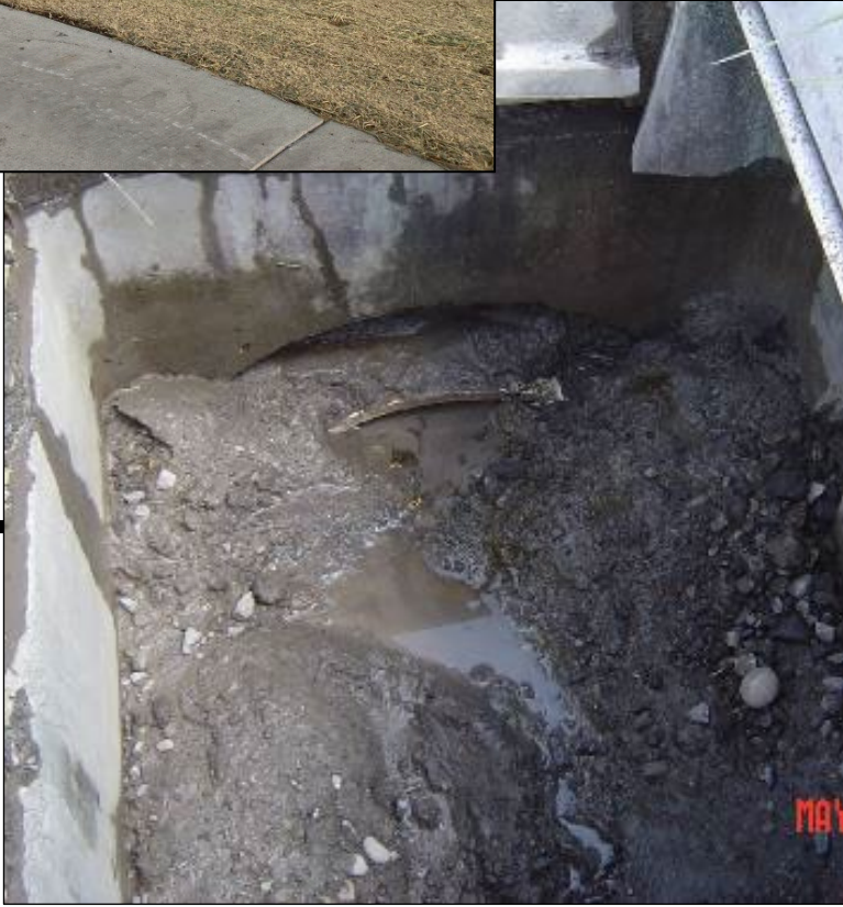
Graphic 5.0.2: Inlet sump clogged with construction debris
