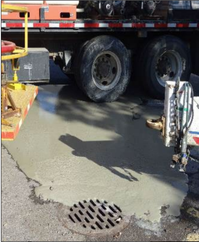
Graphic 4.0.1: Bentonite slurry spill
