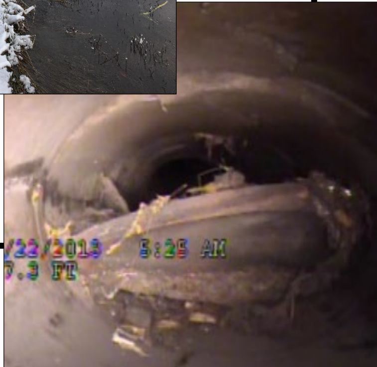
Graphic 1.0.2: Failed stormwater pipe
