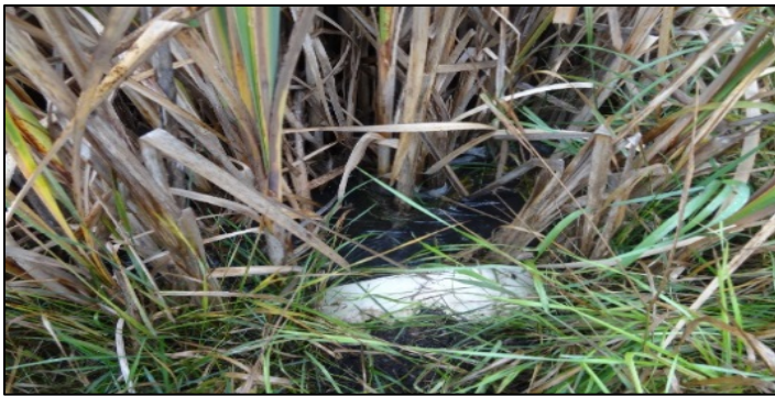
Image 4 - Obstructed inlet pipe
