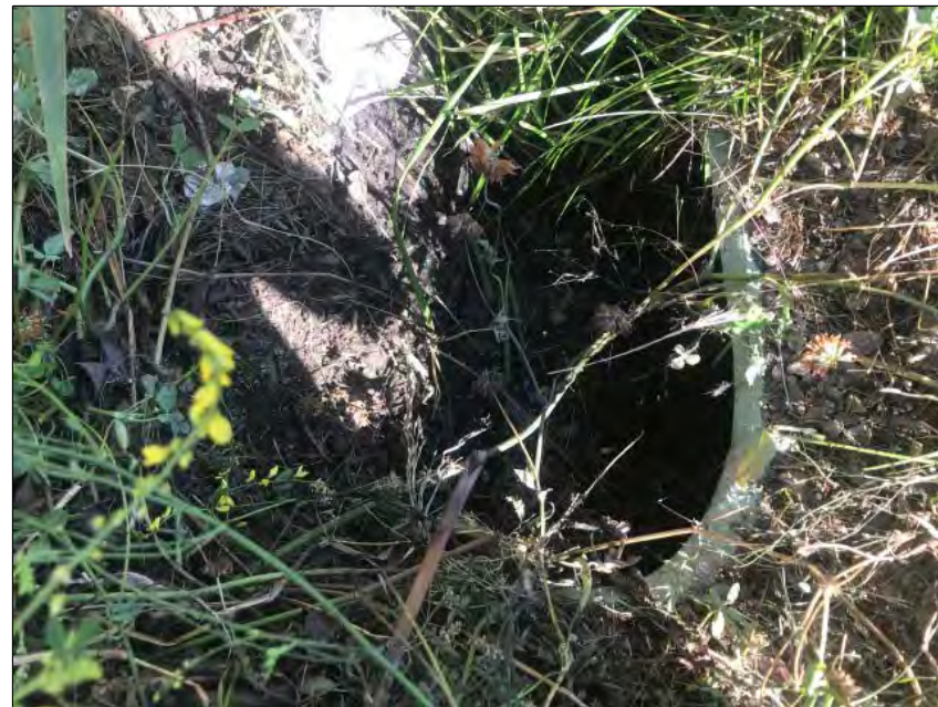
Image 2 Inlet pipe with accumulated sediment.
