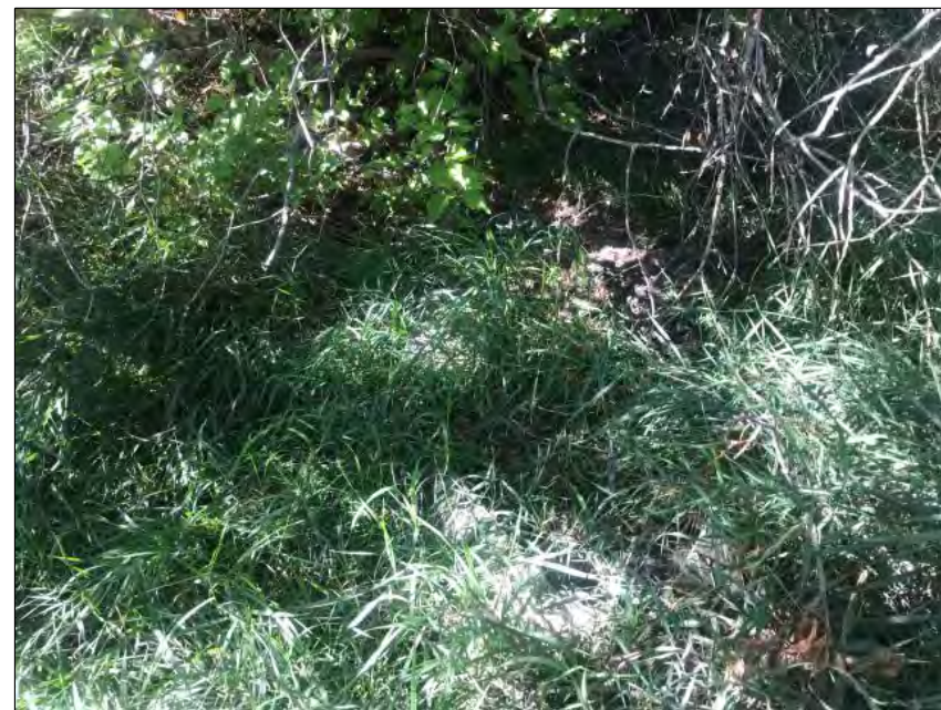
Image 2 Inlet from road CMP; abundance of vegetation clogging structure.
