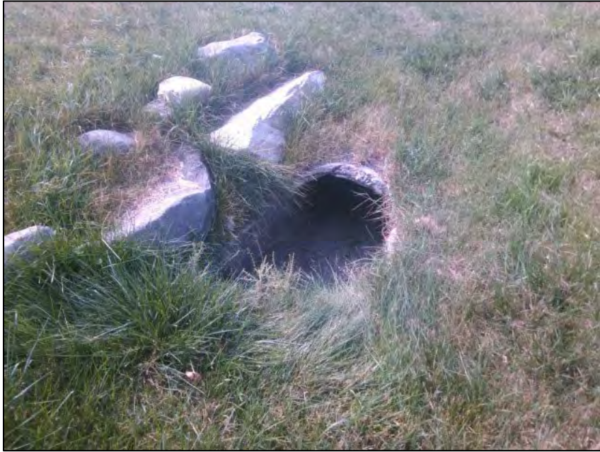
Image 3 Facility inlet/outlet. Small amounts of sediment in pipe.
