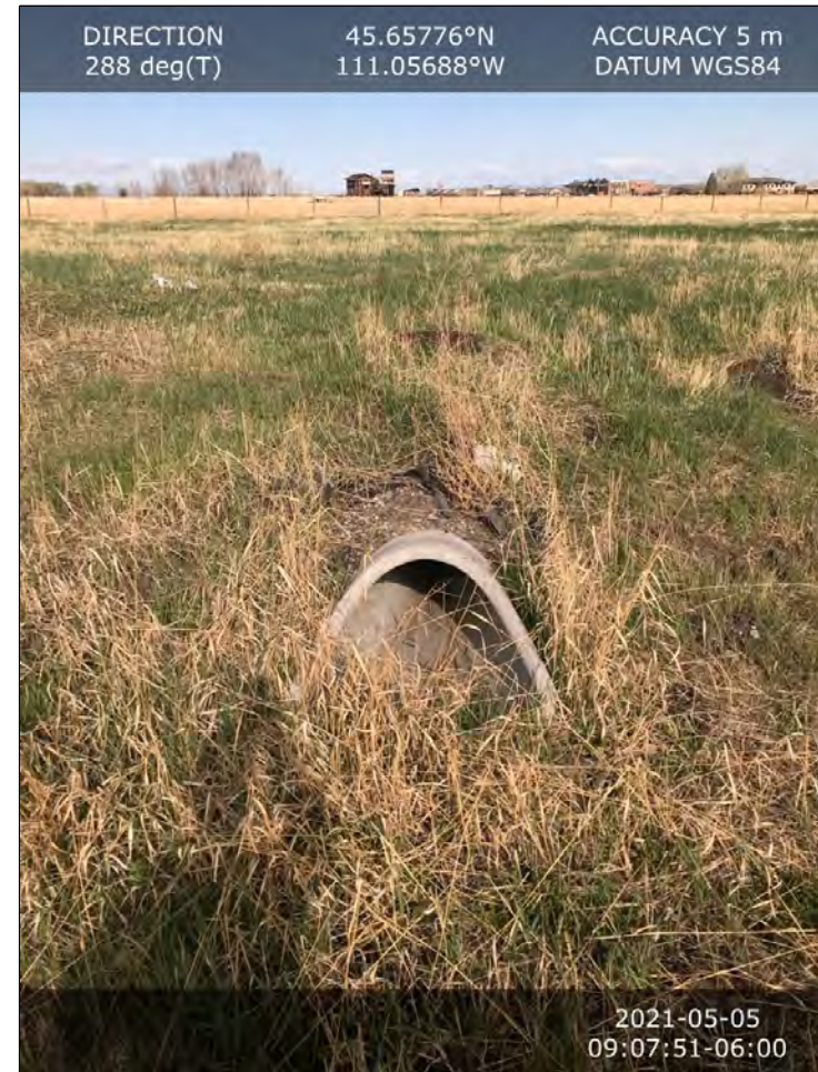
Image 2 Outlet from the facility, outlet structure can be seen about ten feet behind it. (west view)
