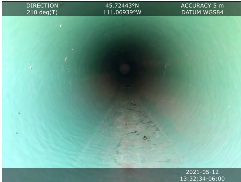
Image 3 PVC outlet from basin to outlet structure. There is no evidence of recent flow. (north view)
