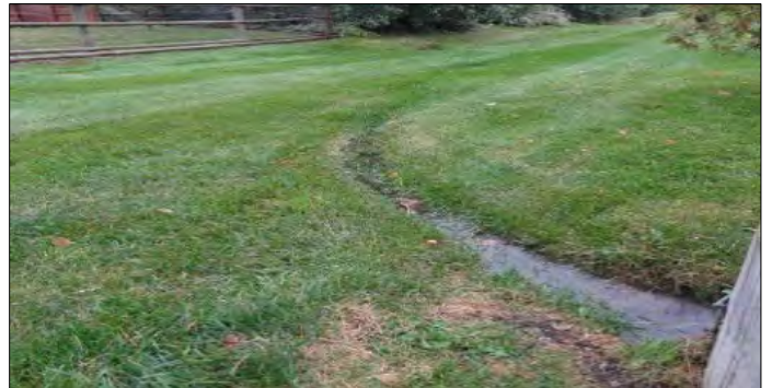
Image 3 - Erosion causing channelized flow
