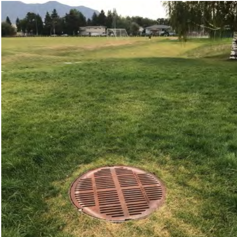
Image 3 Slotted manhole, leads to basin at center of photo. Parking lot drains from curb cut by the birch tree at upper right. (northeast view)
