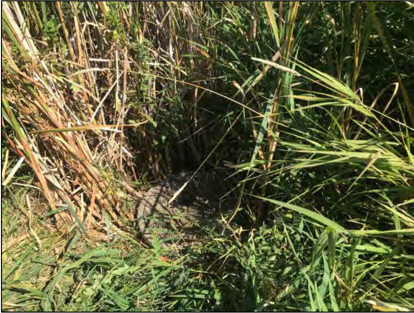
Image 3 Outlet structure; clogged with vegetation.
