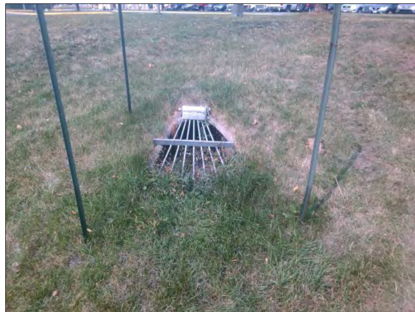
Image 2 Pond inlet (west view). Small amounts of debris and sediment behind trash rack.
