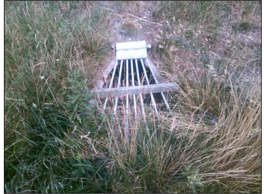
Image 4 Inlet structure (northeast view). Overgrown vegetation.
