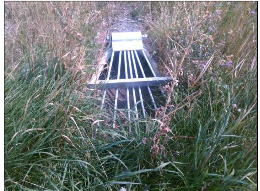
Image 6 Inlet structure facing (northeast view). Overgrown vegetation.
