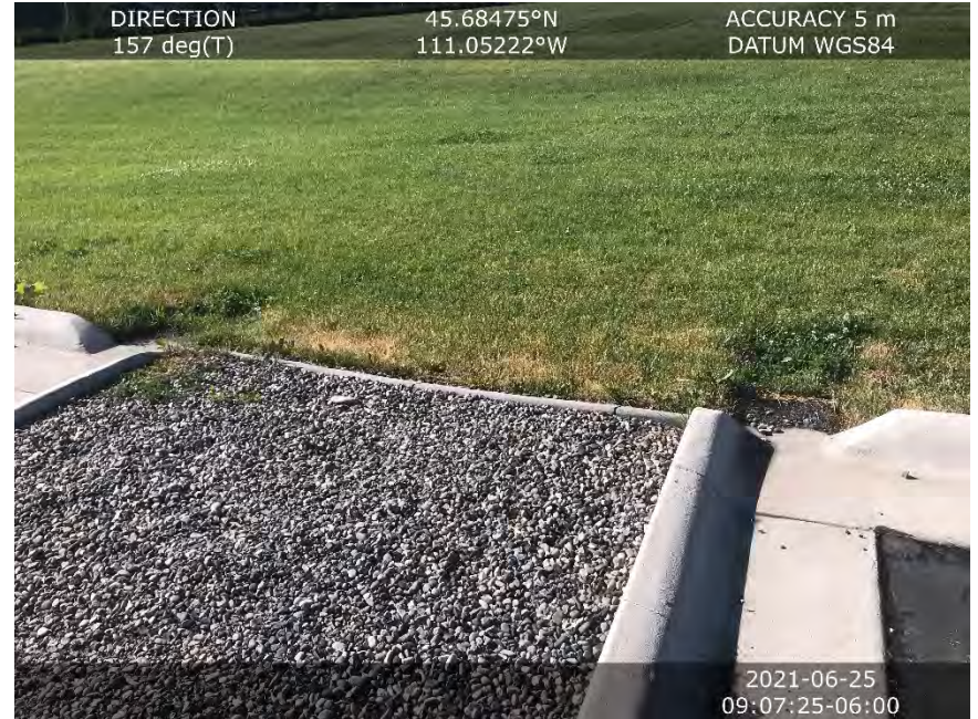
Image 4 Curb cuts leading to facility. This facility also accepts flow from the south and west fields. (south view)
