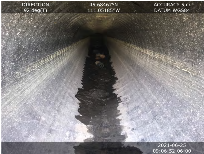
Image 5 Evidence of high flows since last year. Slight debris in outlet structure.
