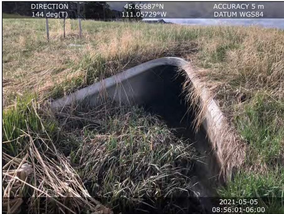
Image 3 Sediment and standing water at facility inlet. (east view)
