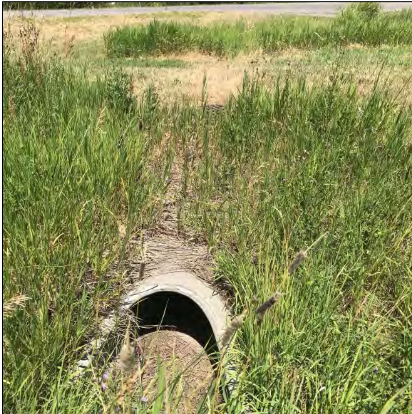
Image 5 Main basin outlet and outlet structure manhole, the control point, visible above center (east view).
