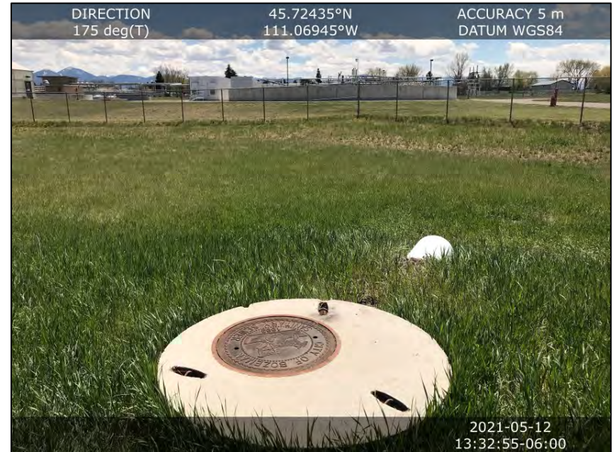
Image 4 Outlet structure and basin. (south view)
