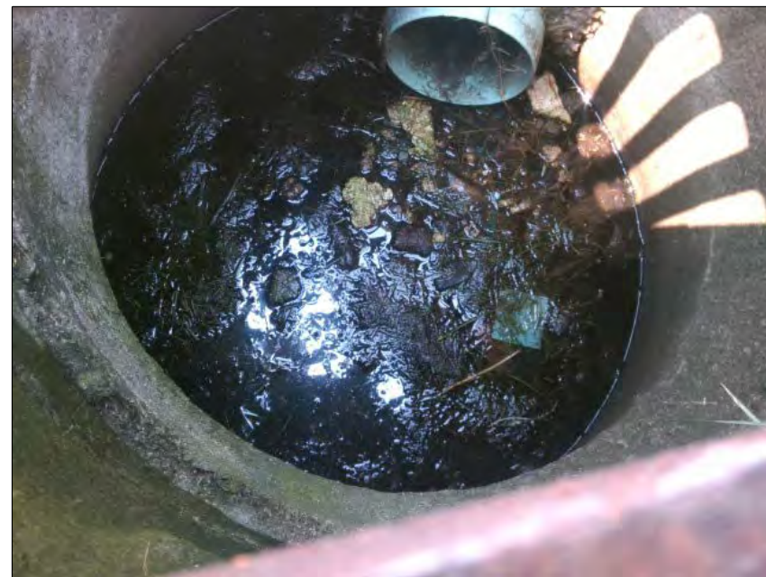
Image 2 Outlet structure sump with debris. (Close-up)
