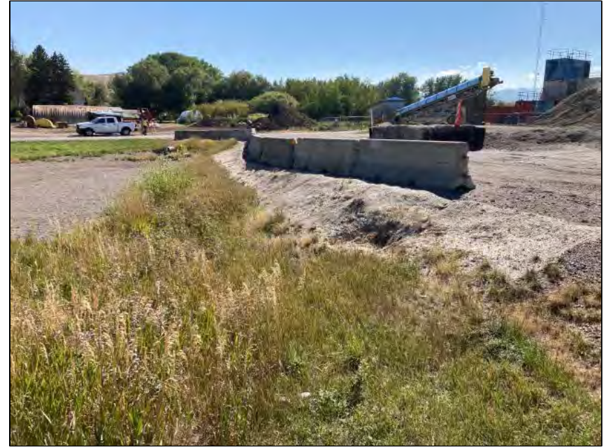
Image 2 Primary detention basin with traction control aggregate facility on right; note concrete barriers and stabilization blanket installed on the break in slope and pond edge, respectively.
