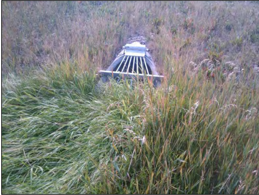
Image 3 Inlet apron (southwest view). Overgrown vegetation.
