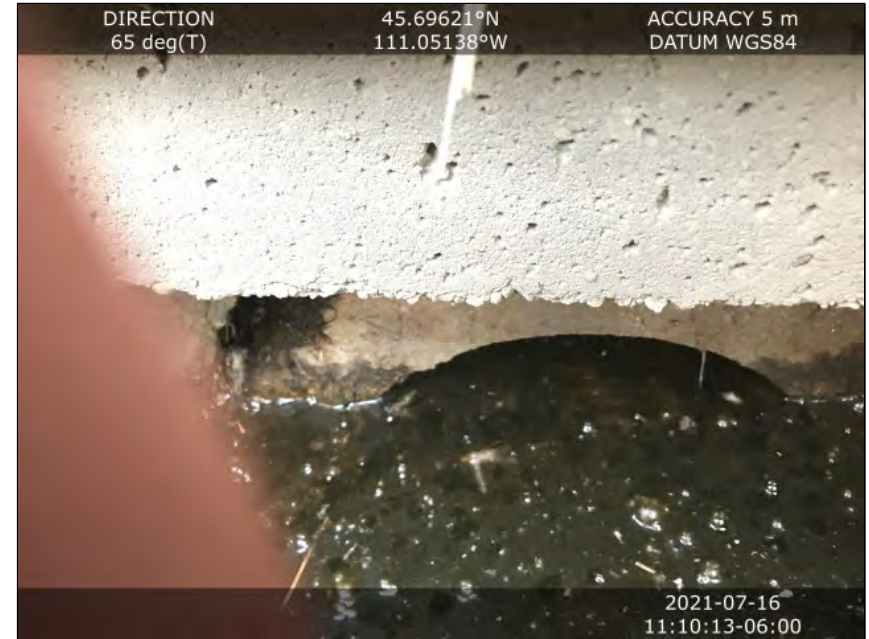
Image 2 Water backed up into inlet structure (close-up view).
