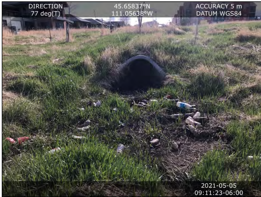
Image 6 Trash and small amount of sediment at facility inlet. (east view)
