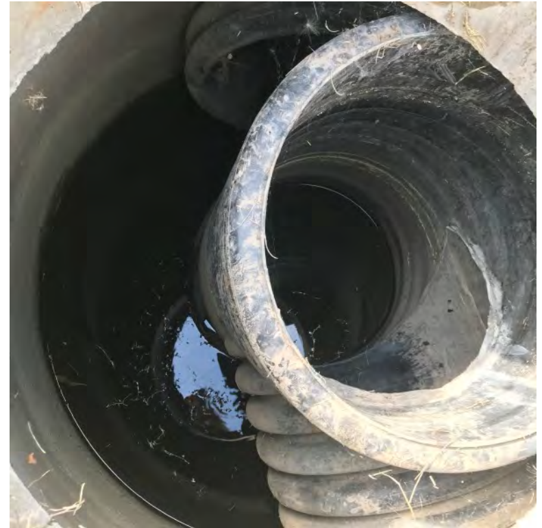
Image 2 Outlet structure. Flow is from top of photo, to tee, bottom of photo to outfall. (close-up)
