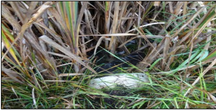
Image 4 - Obstructed inlet pipe
