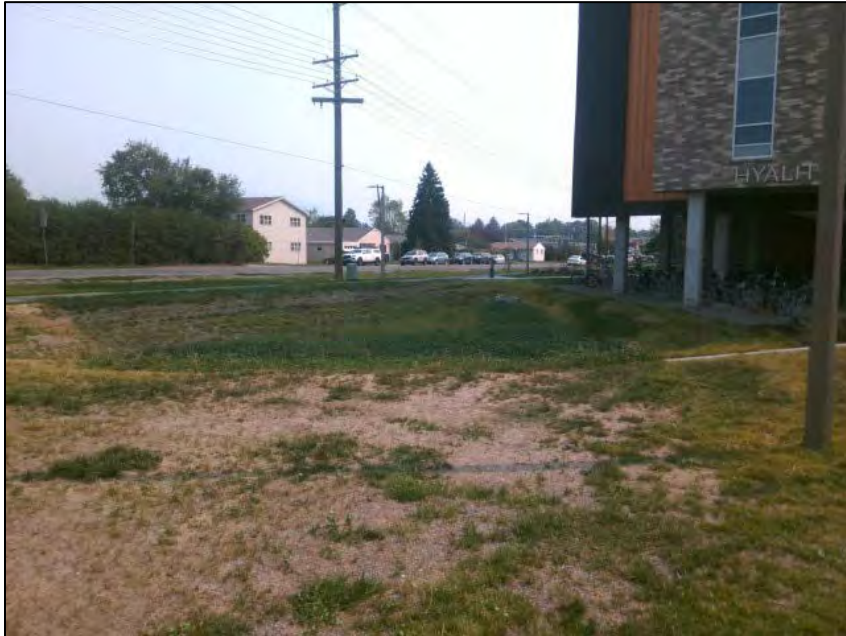
Image 1 Detention pond overview looking (northeast view). Note bare ground on top break.
