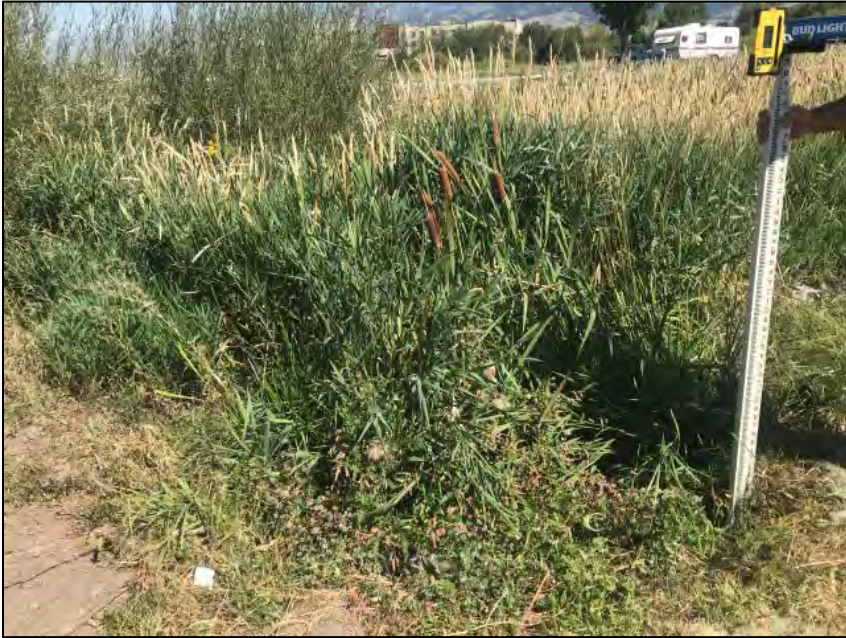
Image 3 Inlet pipe location (at survey stadia); note heavy overgrowth of detention basin.
