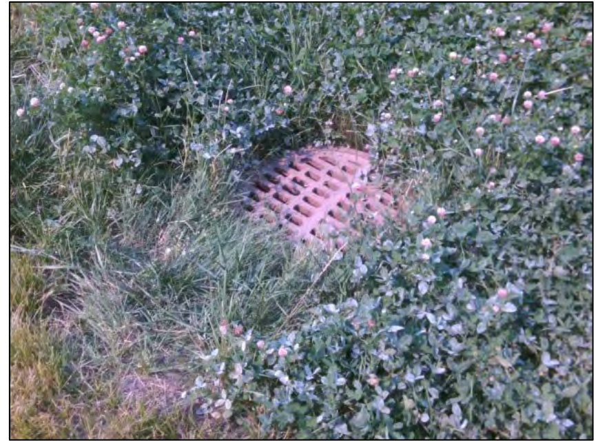
Image 6 Drywell; vertical infiltration drain. Note heavy cover of red clover.
