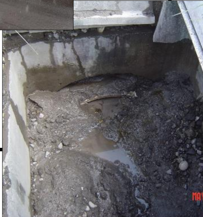
Graphic 5.0.2: Inlet sump clogged with construction debris
