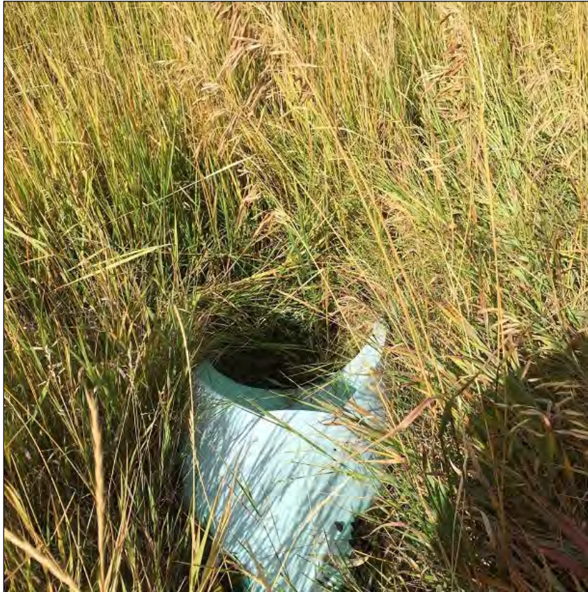
Image 5: Stormwater basin discharge pipe (west view)
