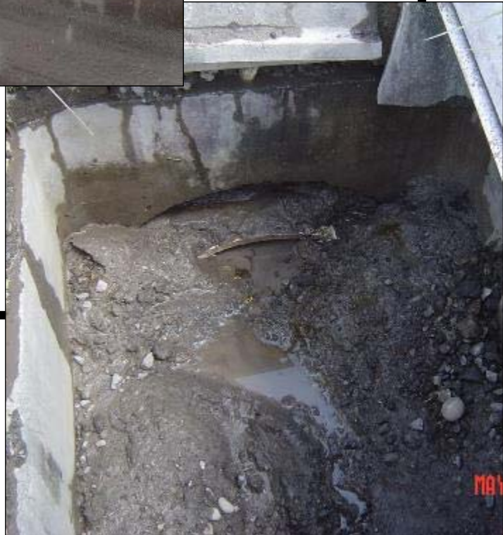
Graphic 5.0.2: Inlet sump clogged with construction debris
