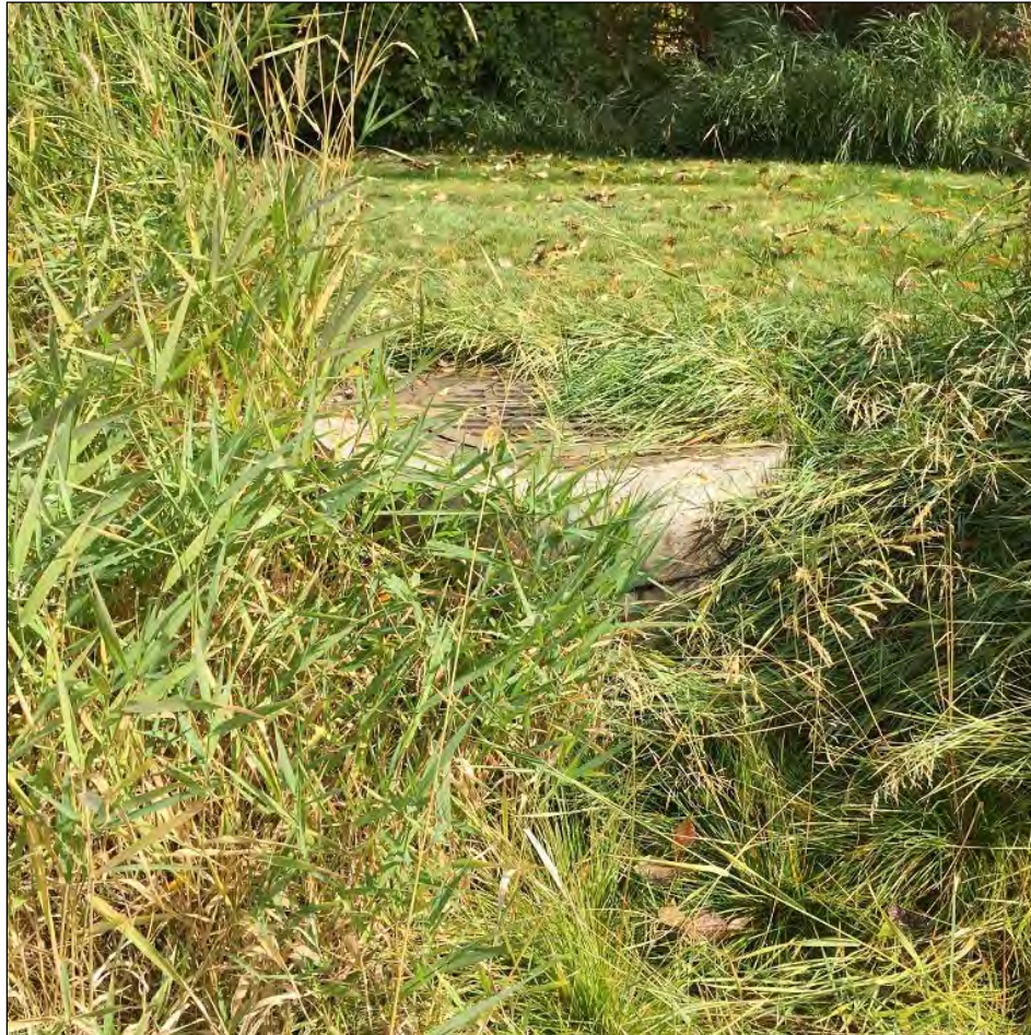
Image 4: Outlet structure overview showing overgrown vegetation (east view)
