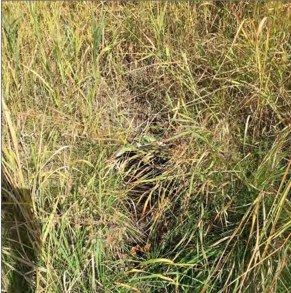
Image 2: Obstructed and clogged inlet pipe (north view)
