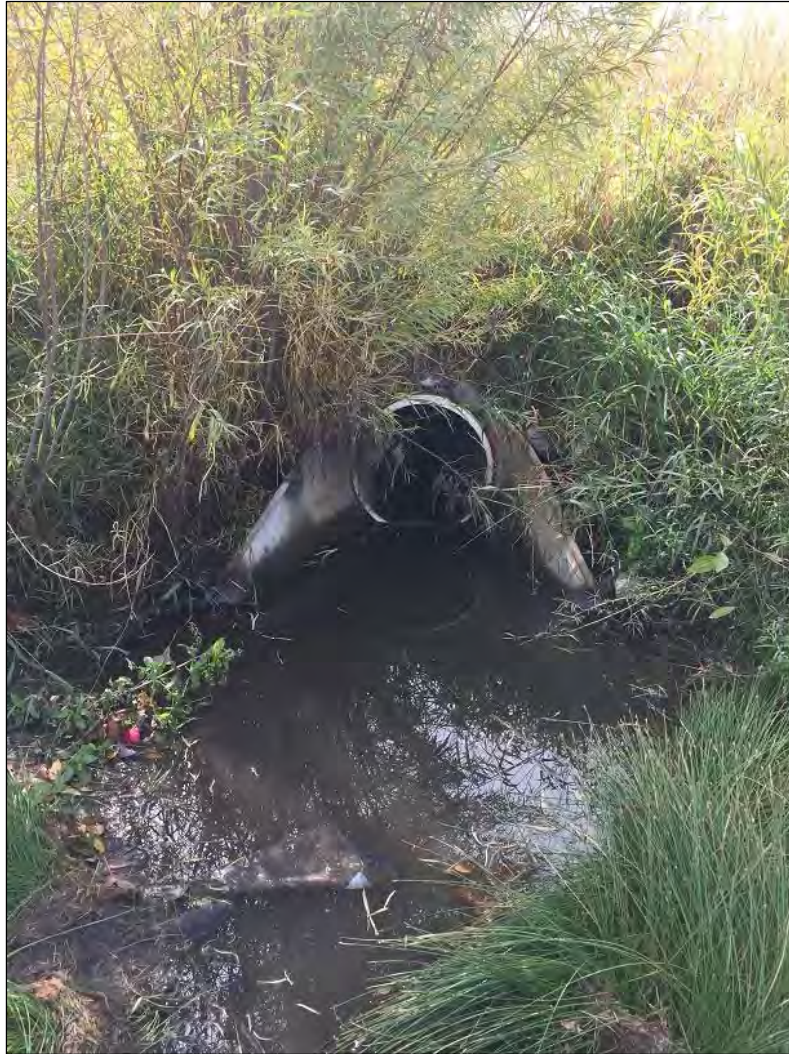
Image 4: Second inlet pipe and accumulated debris (south view)
