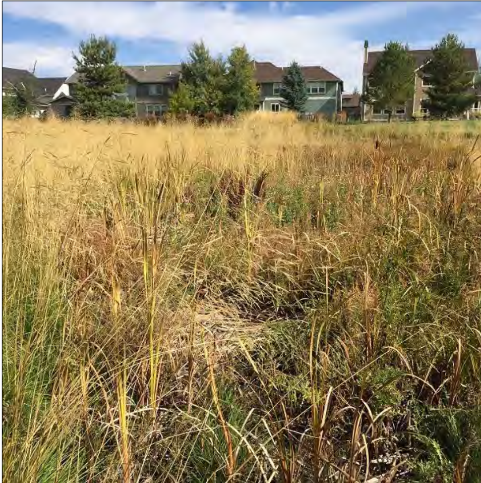
Image 3: Stormwater basin overview showing overgrown vegetation (east view)
