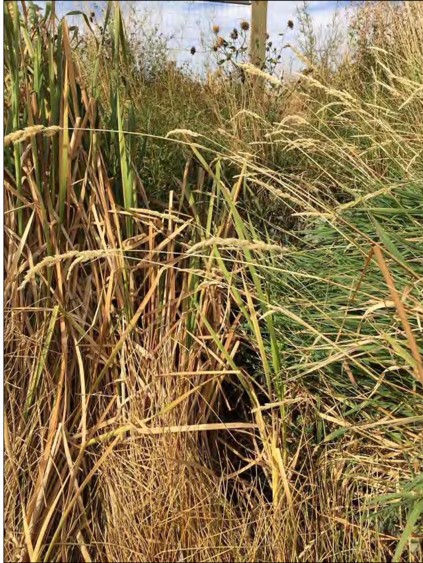
Image 3: Obstructed and clogged inlet pipe (west view)
