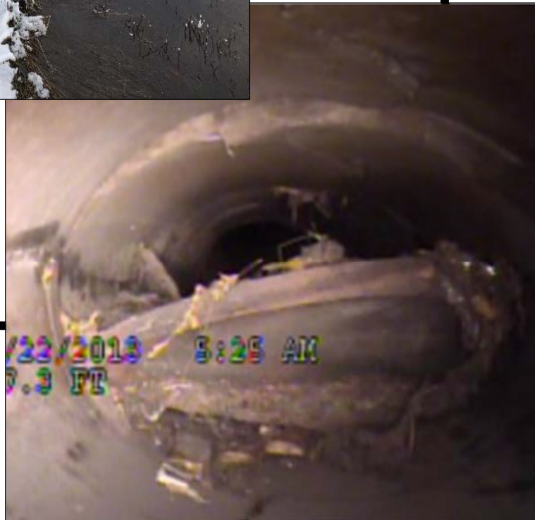
Graphic 1.0.2: Failed stormwater pipe
