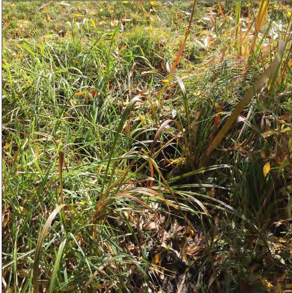
Image 2: Obstructed and clogged inlet pipe (south view)
