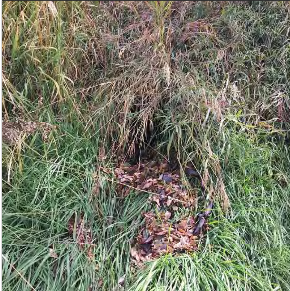
Image 2: Obstructed and clogged inlet pipe (1 of 3)
