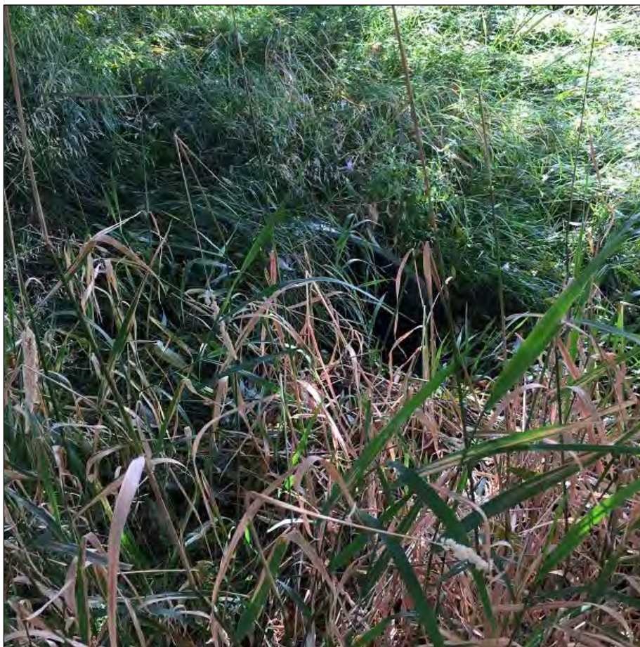
Image 2: Obstructed and clogged inlet pipe (south view)
