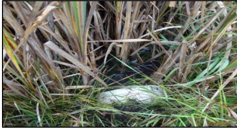
Image 4 - Obstructed inlet pipe
