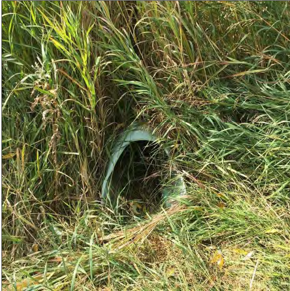
Image 5: Stormwater basin discharge pipe (west view)
