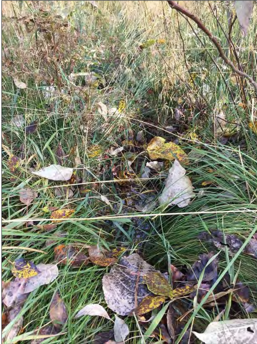
Image 2: Obstructed and clogged inlet pipe (west view)
