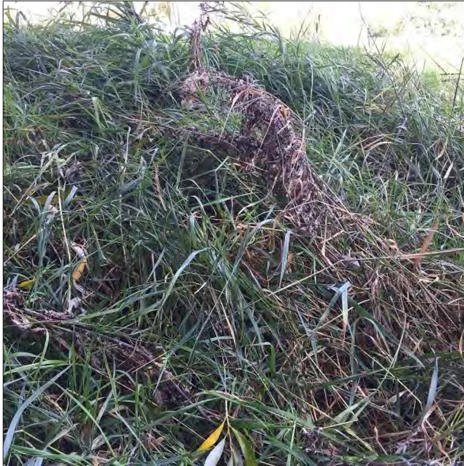
Image 2: Obstructed and clogged inlet pipe (north view)
