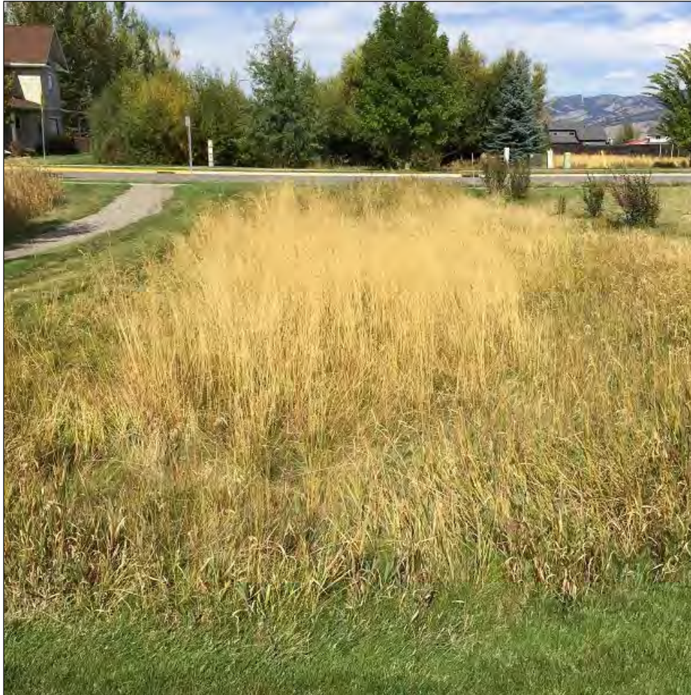
Image 3: Stormwater basin overview showing overgrown vegetation (north view)
