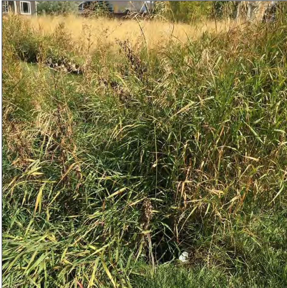
Image 5: Clogged and obstructed inlet pipe (2 of 3)
