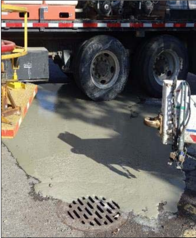
Graphic 4.0.1: Bentonite slurry spill
