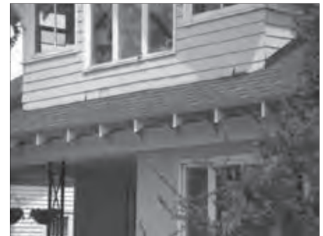
This detail shows ornate rafters which should be preserved during a rehabilitation process.
