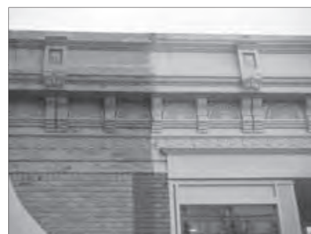
Details such as these should be preserved in order to avoid the need for replacement in the future.
