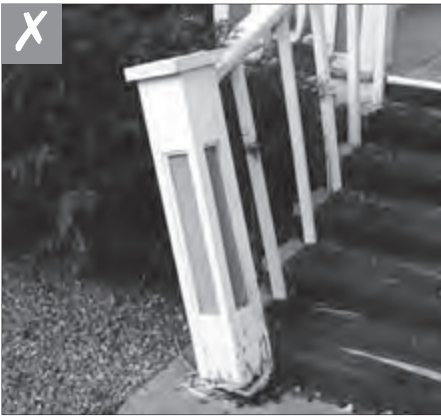
Before: A deteriorated railing should be repaired, rather than replaced.
