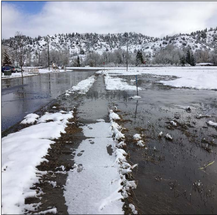
Graphic 1.0.1: Street-flooding resulting from clogged infrastructure
