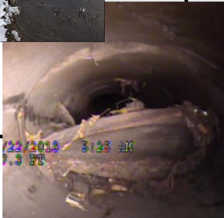
Graphic 1.0.2: Failed stormwater pipe
