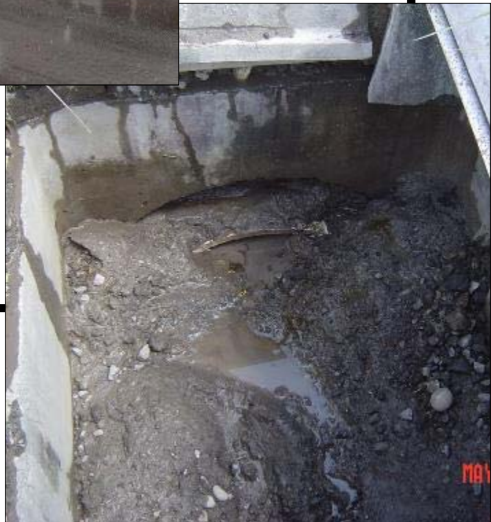
Graphic 5.0.2: Inlet sump clogged with construction debris
